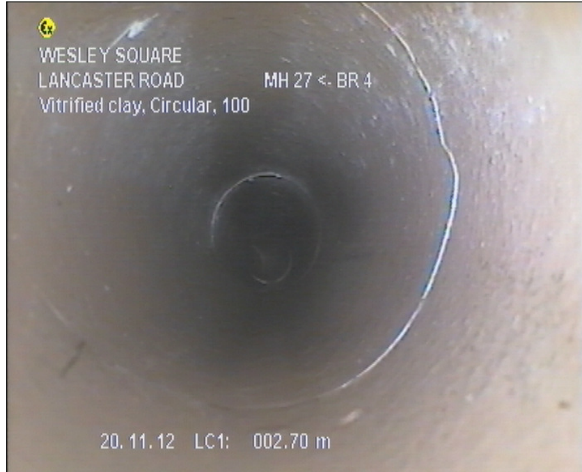
Photo: 538_5a 2.7m, Circumferential Crack, from 11 to 08 o'clock
