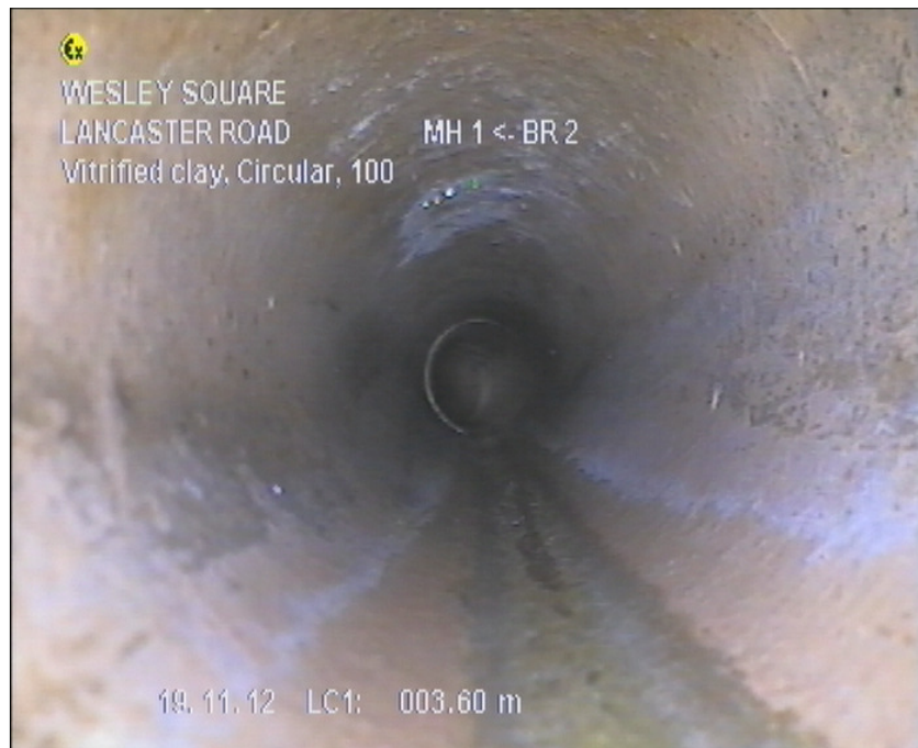
Photo: 2_4a 3.6m, Circumferential Crack, from 12 to 12 o'clock
