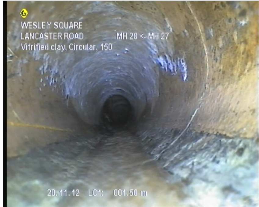
Photo: 84_5A 1.5m, Circumferential Crack, from 12 to 12 o'clock
