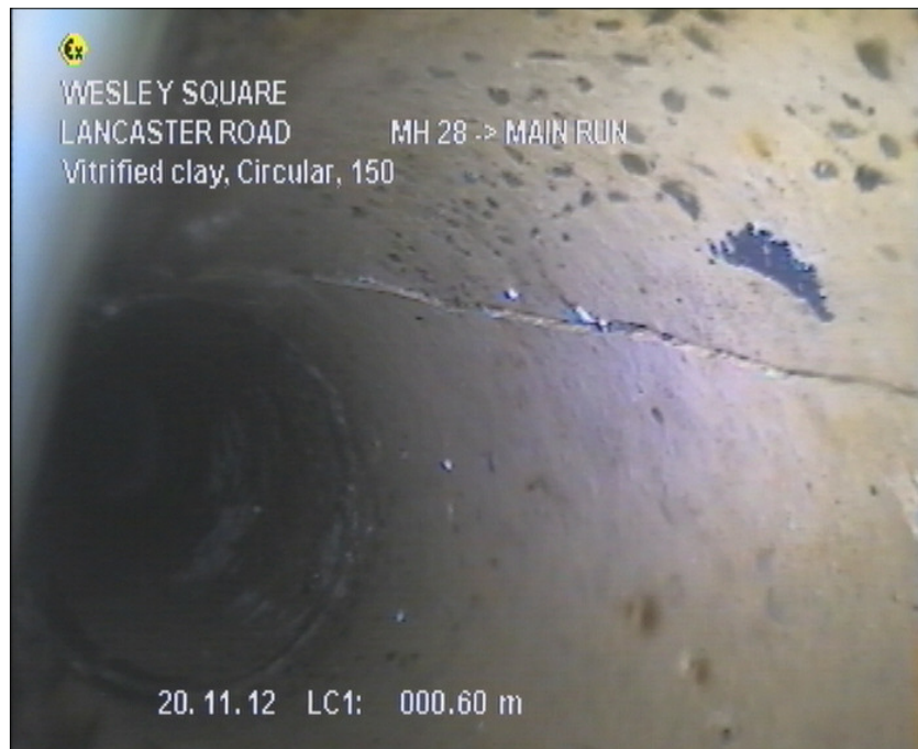
Photo: 86_5a 1.3m, Longitudinal Fracture at 12 o'clock
