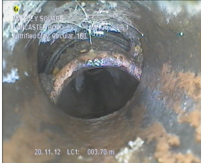
Photo: 492_4a 3.7m, Joint displaced. Large
