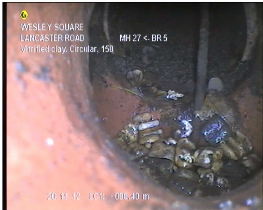
Photo: 79_5A 1.3m, Debris, 20 % cross-sectional area loss
