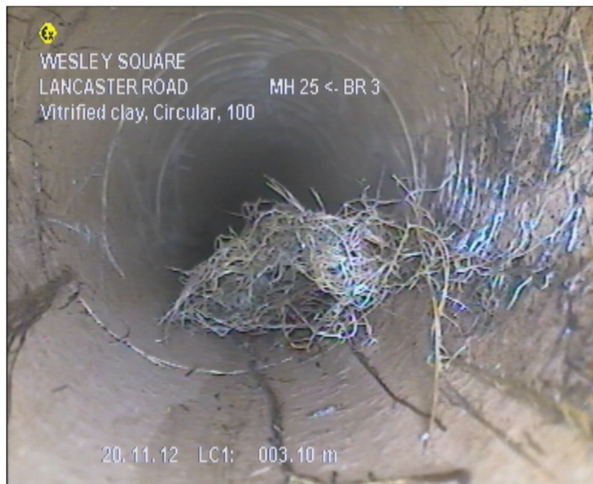
Photo: 483_5a 3.1m, Circumferential Crack, from 12 to 12 o'clock Remarks: SPIRALS
