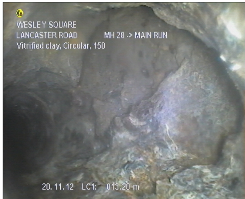
Photo: 599_7a 13.2m, General Observation Remarks: POSSIBLE DISUSED FILLED IN MH
