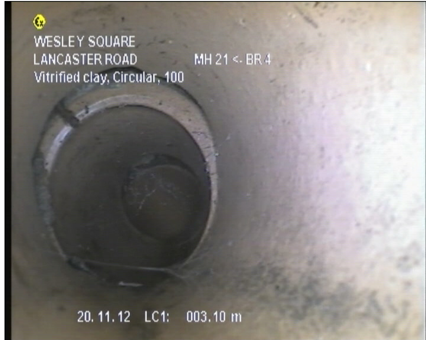
Photo: 65_6A 3.1 m, Joint displaced. Large
