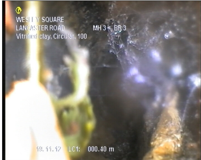
Photo: 7_4A 0.4m, Debris, 40 % cross-sectional area loss
