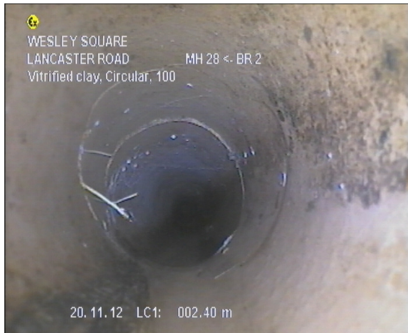
Photo: 559_4a 2.4m, Circumferential Fracture, from 12 to 12 o'clock
