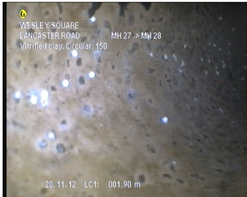
Photo: 55_6A 2.4m, Debris, 20 % cross-sectional area loss
