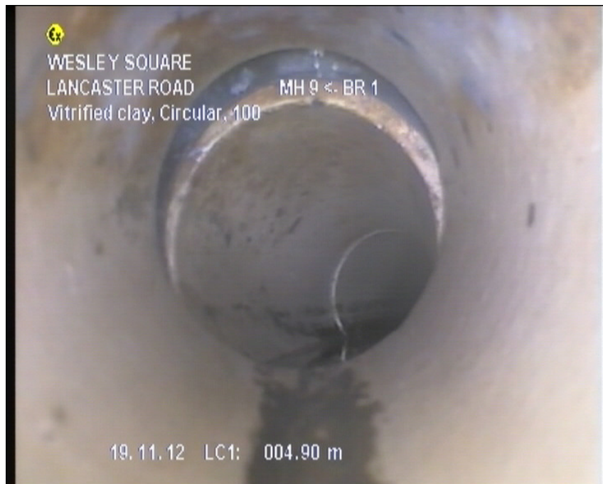
Photo: 35_5A 4.9m, Joint displaced. Medium
