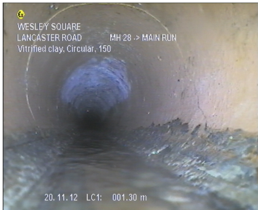
Photo: 86_6a 1.3m, Circumferential Fracture, from 12 to 12 o'clock
