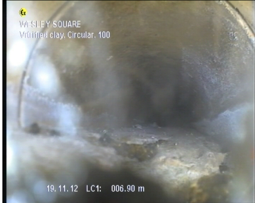
Photo: 43_6A 6.9m, Debris, 30 % cross-sectional area loss
