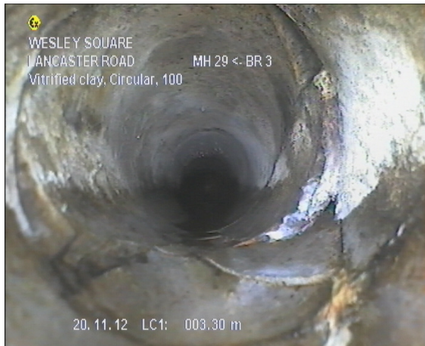
Photo: 629_4a 3.3m, Multiple Fractures from 12 to 12 o'clock
