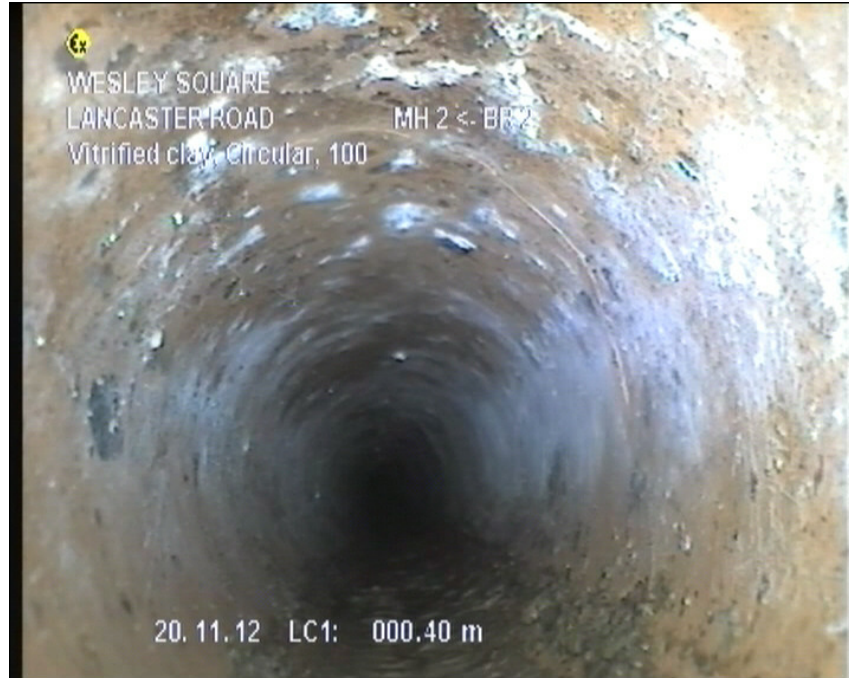
Photo: 46_5A 0.4m, Circumferential Crack, from 10 to 03 o'clock
