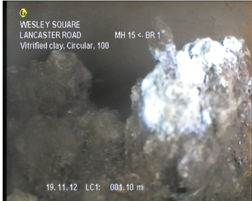
Photo: 38_4A 1.1m, Debris, 70 % cross-sectional area loss
