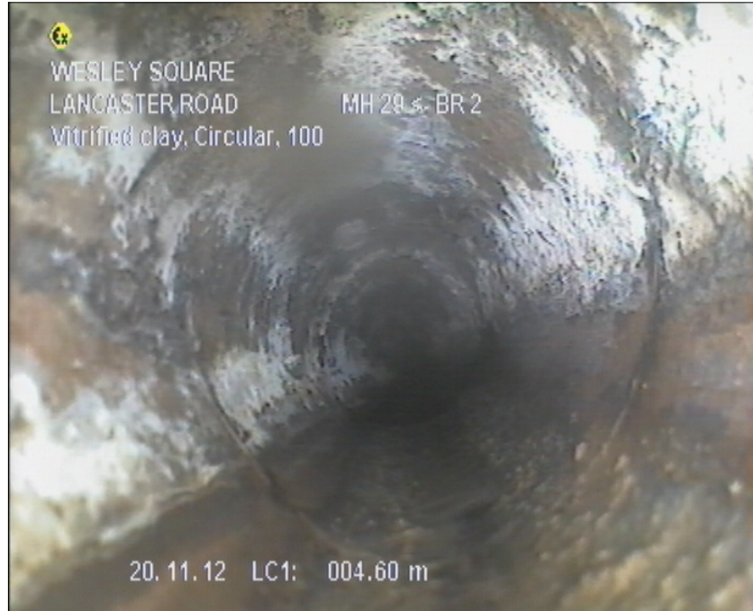
Photo: 621_5a 4.6m, Circumferential Crack, from 12 to 12 o'clock
